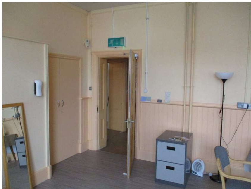
Photo 21 – Restricted access adjacent leading edge to classroom door.
