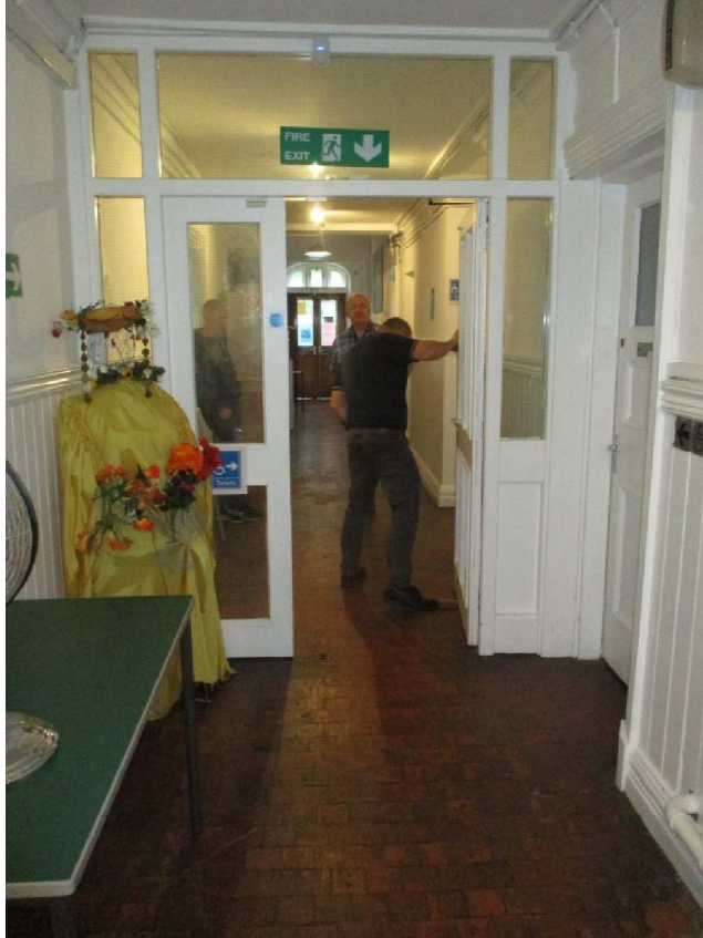
Photo 12 – Cross corridor door, not held open.
